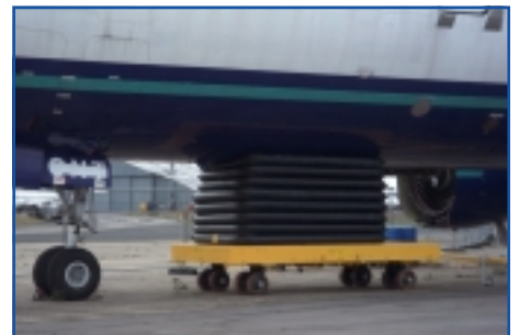
Nose lift of a DC10 aircraft. 30 tonne Single element airbags were used for the lift, they also acted as a cushion to prevent damage to the aircraft skin.
