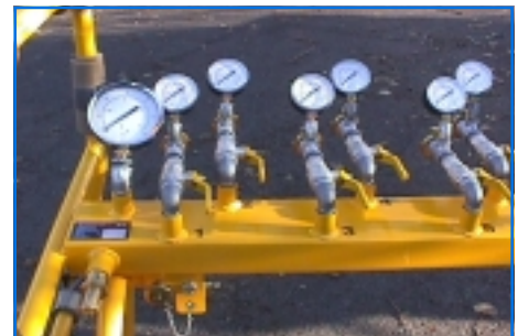
Control Valves and Pressure Gauges on Console 10001-20
